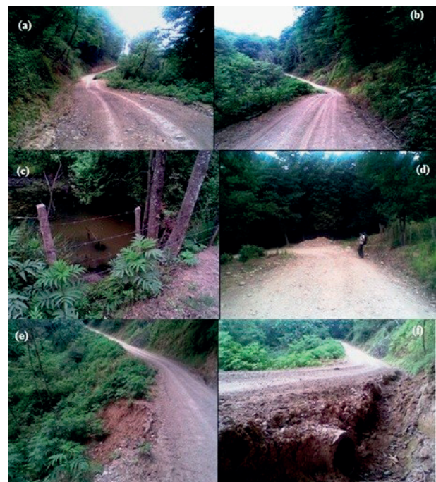
Figure 4. Effect of vertical and horizontal curves on locating culverts (A, B); accumulation of water due to the absence of culvert and ditch (C); effect of horizontal curve, superelevation as well as suitable interval between culverts on locating culverts (D); landslide occurrence due to the absence of drainage systems; improper installation of culvert (F)
