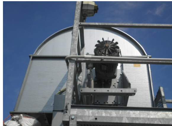
Fig. 9. Drive of bucket elevator (electric motor without cover)
