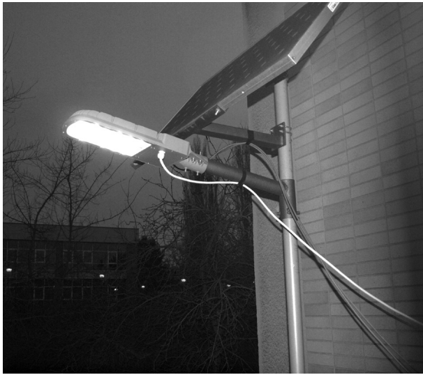
Fig. 1. Outdoor section of the off-grid PV system
