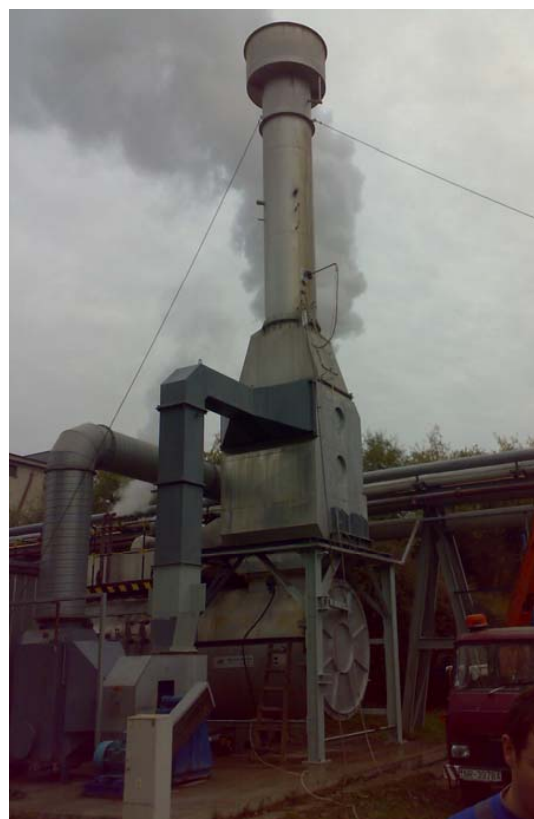
Fig. 5. Data sampling – tested thermal deodorising oxidiser
