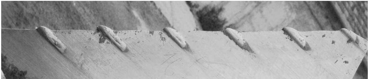
Fig. 4. Detailed view on wear course at oblique overlays after ploughing 18 ha, added material OK Tubrodur 14.70
